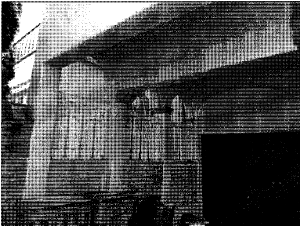
Figure 21. Detail of perimeter wall at east boundary, ceiling in front of garage and garage door, view southeast (SWCA, 2018).
