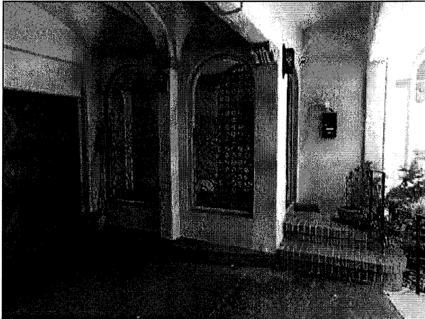
Figure 19. Detail of side entry at the junction of the two volumes, view west (SWCA, 2018).
