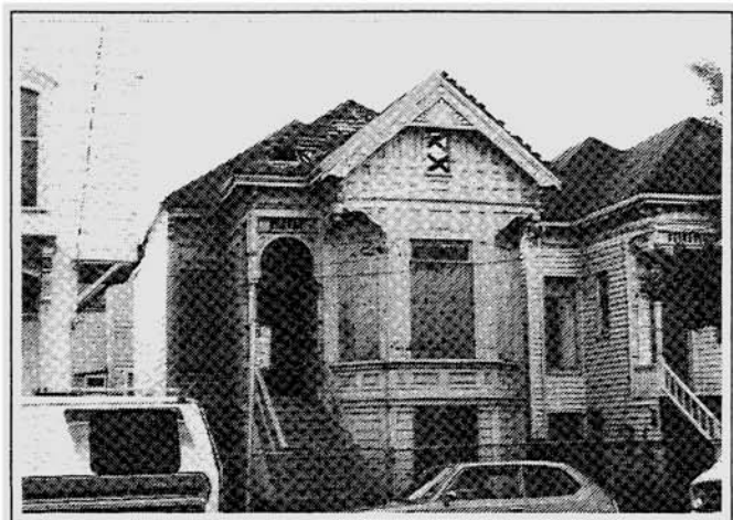
Owner-installed building security measures which the City has considered acceptable are often ineffective, create blight, and attract vandals, arsonists and other criminals.
