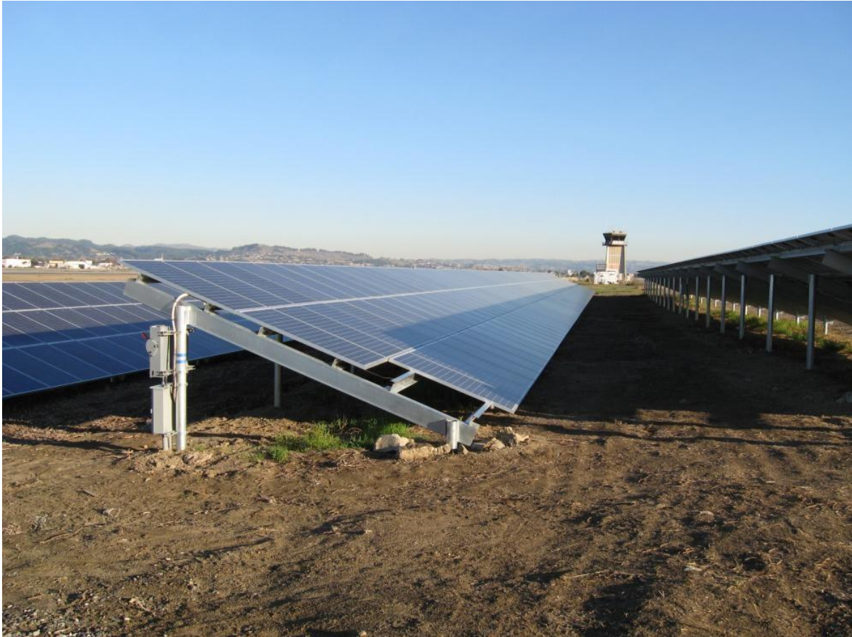
Above: A portion of the solar array located at the Oakland International Airport.
