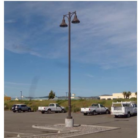
Example of freestanding light fixture in parking area
