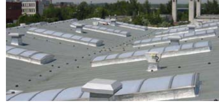
Example of roof penetrations (vents and skylights) arranged in an organized, repetitive design
