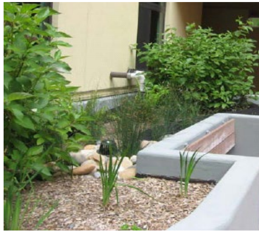
Figure 8-15. The same planter as shown in Figure 8-14, after vegetation has matured and partially conceals the half-buried pipe from view.
