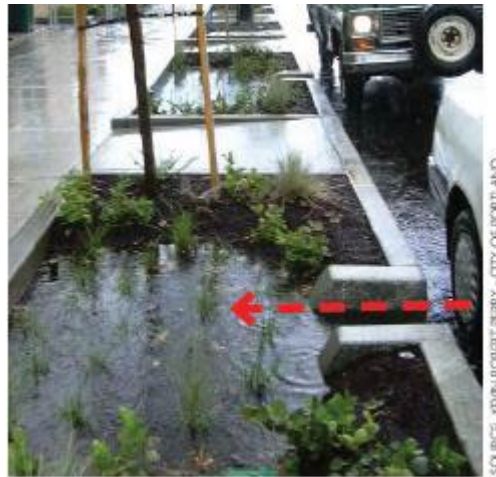
Figure 7-10. The side wings of this standard curb cut help retain the side slope grade on each side of the curb cut opening.
