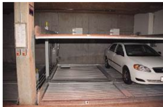
Figure 5-5. Parking Lifts in Parking Garage, Berkeley
