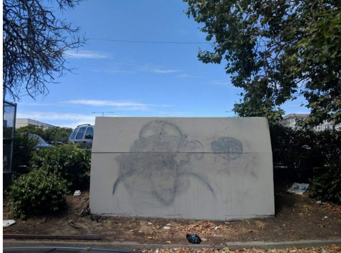
VENT: TO REMAIN FINAL DESIGN TREATMENT TO BE DEVELOPED WITH BART. OPPORTUNITY FOR ART.
