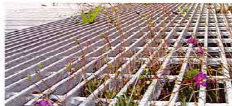
METAL GRATE LID AT BIORETENTION BASIN
